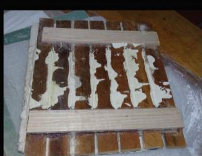
Keys are Rebuilt to Adhere the 130 Year Old Plaster to the Lath
