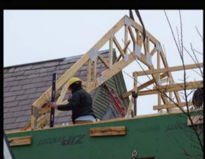
The Roof was Designed to be Removed in it's Entirety With One Crane Pick
