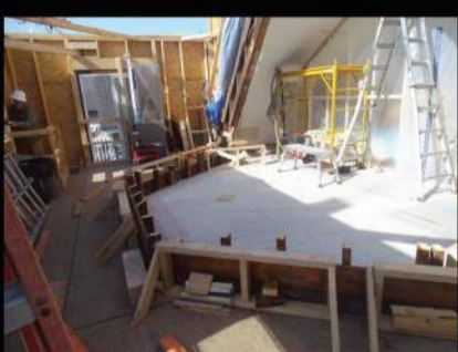
After the Mural is Cut From the Integrated Roof Structure & Building Side Walls
